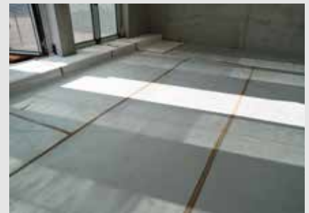
The non protected window is creating glare.
